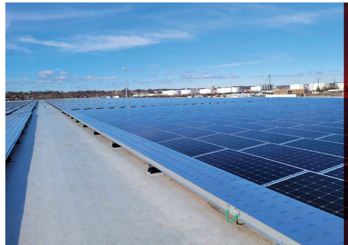
Perth Amboy Community Solar Project. 2020. Image courtesy of New Jersey's Clean Energy Program.
